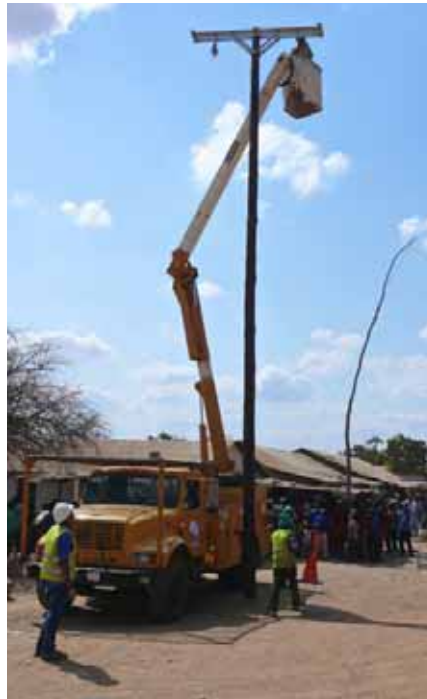
Pike workers install medium-voltage wire, which will supply electricity to Chamae Village for the first time.
